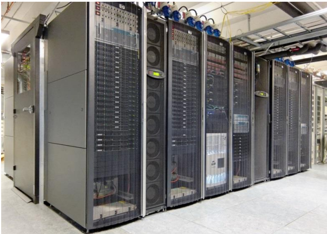
Complete system designed and built by Starfish Technologies
